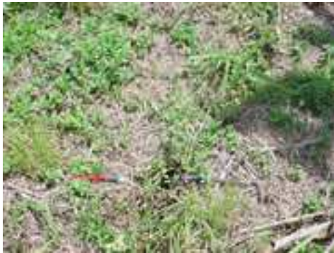
Photo 12: The ground developed cracks in dry season. Surface cracks are indicators of soil that is prone to swelling and shrinking. The width of the cracks is as much as 6”
