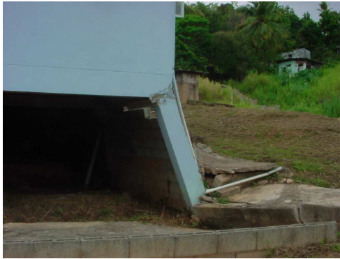
Photo 1: The house got damaged because of land slip towards right side.
