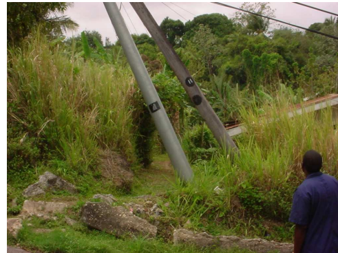
Photo 4: Debris of the retaining wall and the bent electrical poles.
