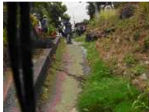
Photo 6: This road has been damaged. Soil moved on to the road.
