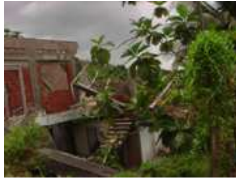
Photo 2: Part of the house towards the observer was damaged
